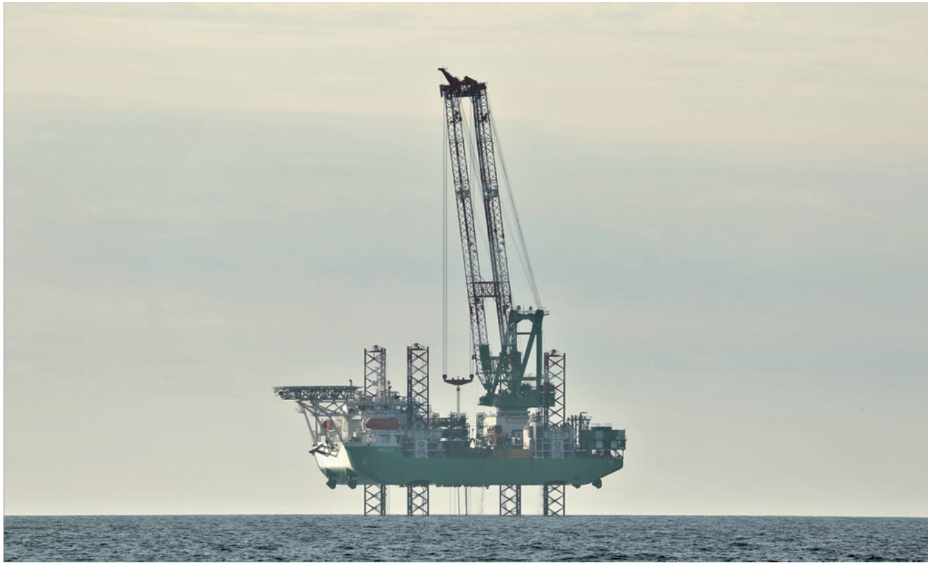
Figure 1: A jack-up pile driving vessel installing wind turbine foundation piles in the Moray Firth, July 2019 © University of Aberdeen.
